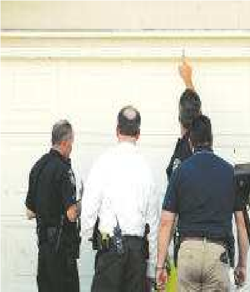
Vacaville police officers on Monday examine a bullet hole above the garage of a home in the 100 block of Rocky Hill Road. (Joel Rosenbaum)
